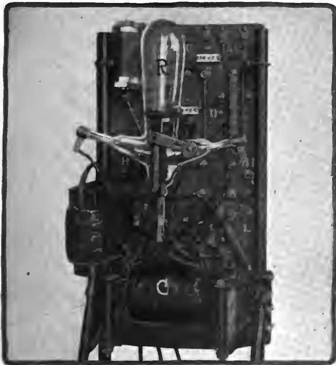
Fig. 3—Swivel-mounting of mercury bulb behind panel of General Electric Company's rectifier
